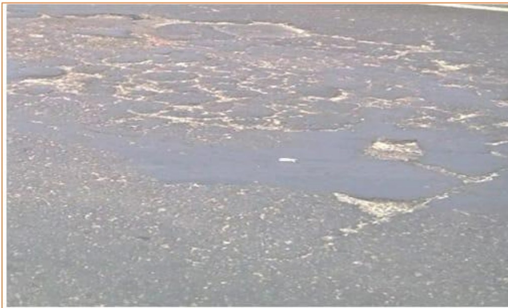
Figure: Block cracking at Chatta meel
