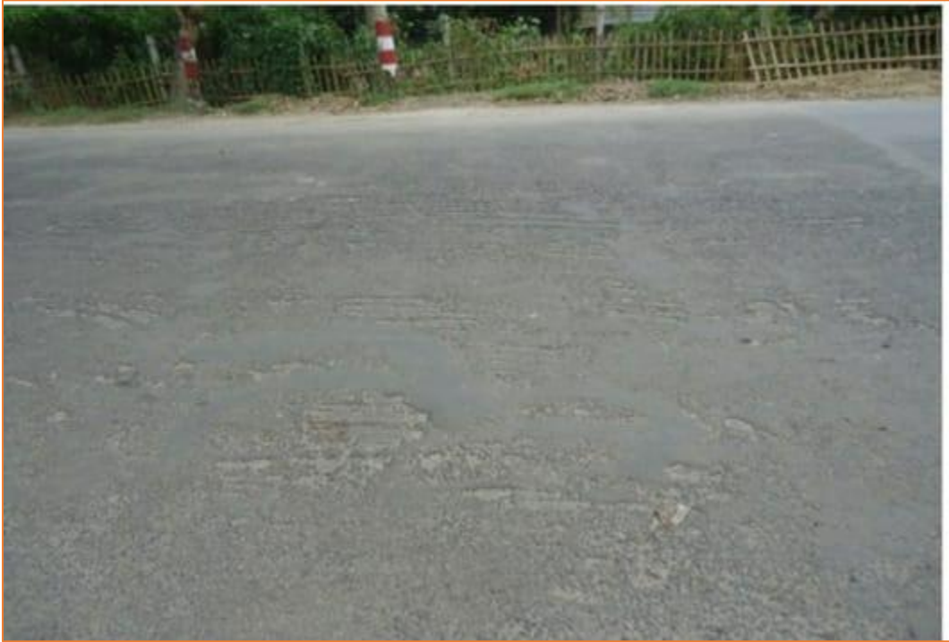
Figure: Slippage cracking at IIM
