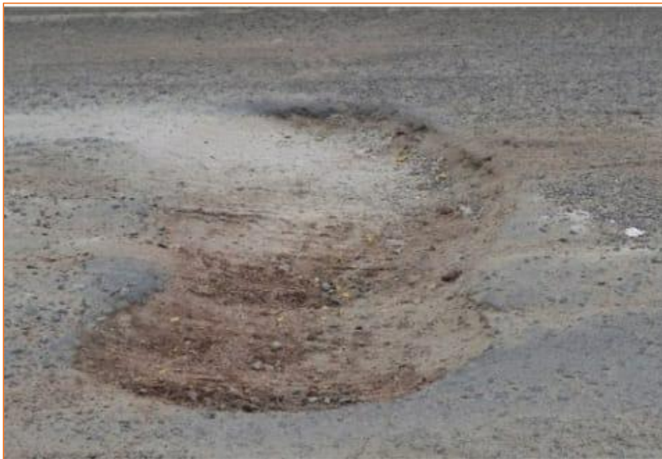
Figure: Potholes at Tadikhana
