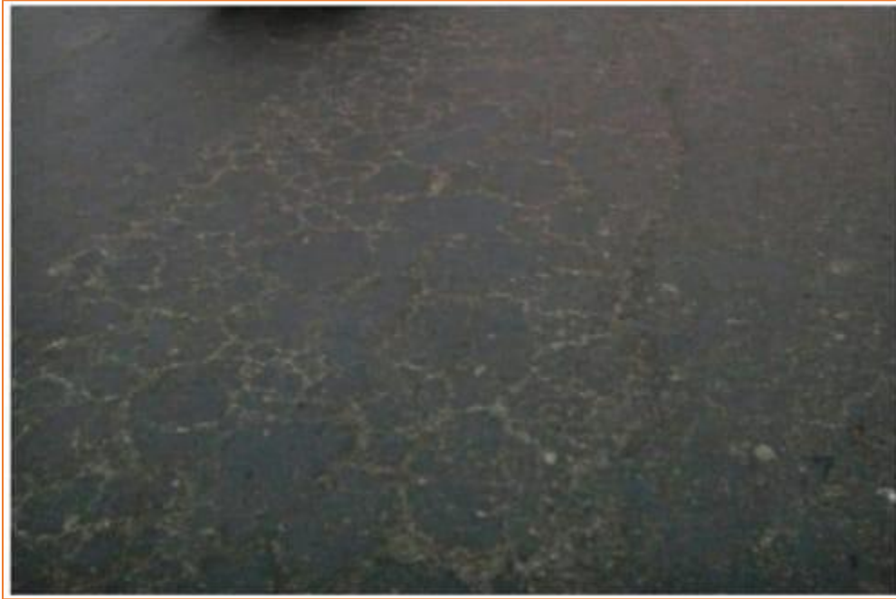
Figure: Alligator cracking at Bkt
