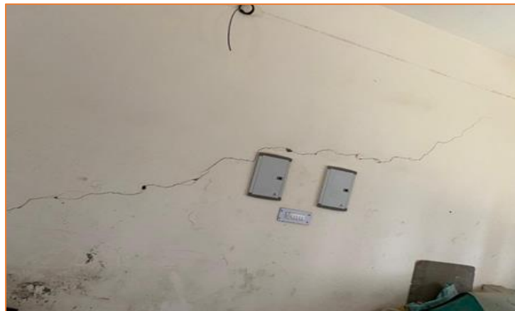
Figure 2: Cracks on walls
