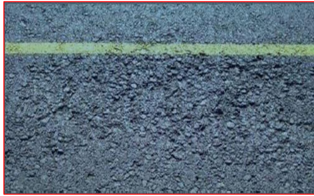
Figure: Segregation of Coarse Aggregate
